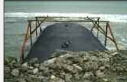
Geotube® unit being held in place by steel frame as it is filled.
